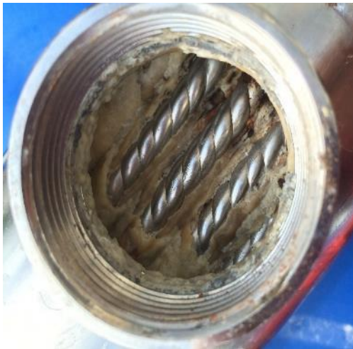
Fig.1. Flow heat exchanger inlet, covered mostly with calcium carbonate scale.
