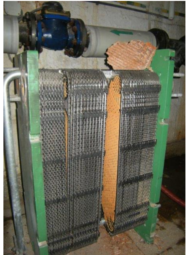
Fig. 3. Demountable flat heat exchanger covered mostly with calcium carbonate scale
