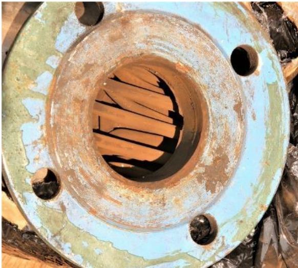
Fig. 6. JAD 6/50 flow HE inlet from DHW system, scaled with calcium and iron compounds.
