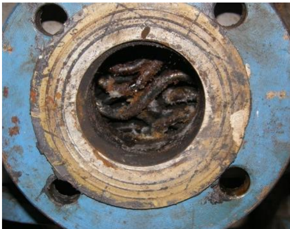
Fig.2. Flow heat exchanger inlet, covered mostly with the scale containing mostly iron compounds.
