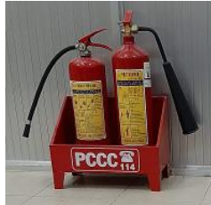
(a) Landmark image with two red fire extinguishers
